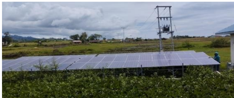
Figure 2: Solar Power Plant
